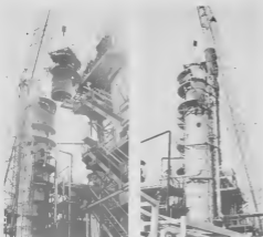
As one of the major activities in the recent Pipestill No. 5 turnaround, 16 feet of the Kero Stripper was replaced for a new section.
